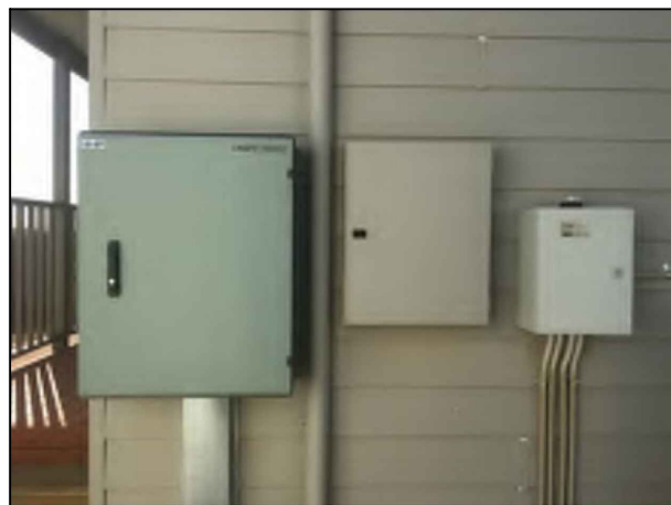
PHOTO 3 (POWER DISTRIBUTION BOARD)
