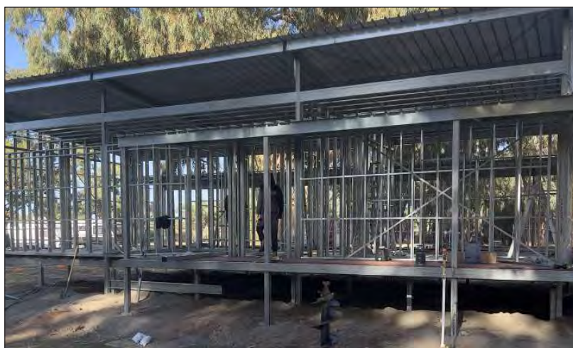
The new amenities block, for Victory Caravan Park, Wilcannia, was designed in accordance with disability access requirements. Picture of works- May 2023.
