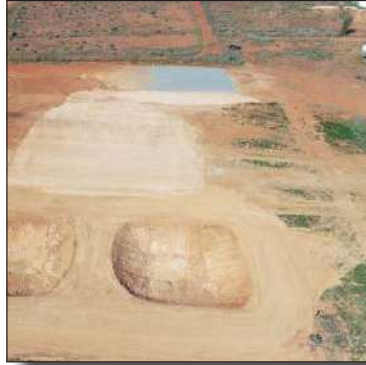
Works commenced at the new White Cliffs Water Treatment Plant Site but are now on hold.
