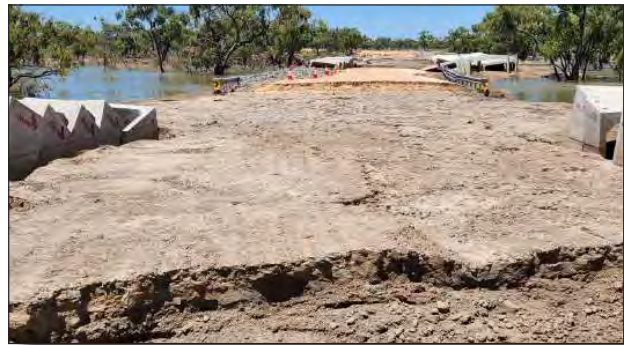
Massive damage to road infrastructure at Menindee 2023.
