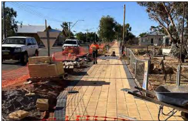
Pictured left, pavement work conducted during the year outside the White Cliffs Public School.
