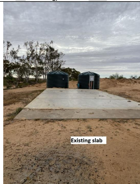
Figure 3: Remnant slab from former camp kitchen to be repurposes and incorporated into new structure (water tanks north facing)
