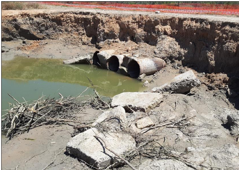
This image was taken on February 4, 2023. The extent of the damage is widespread in the Shire and the work ahead will take time.
